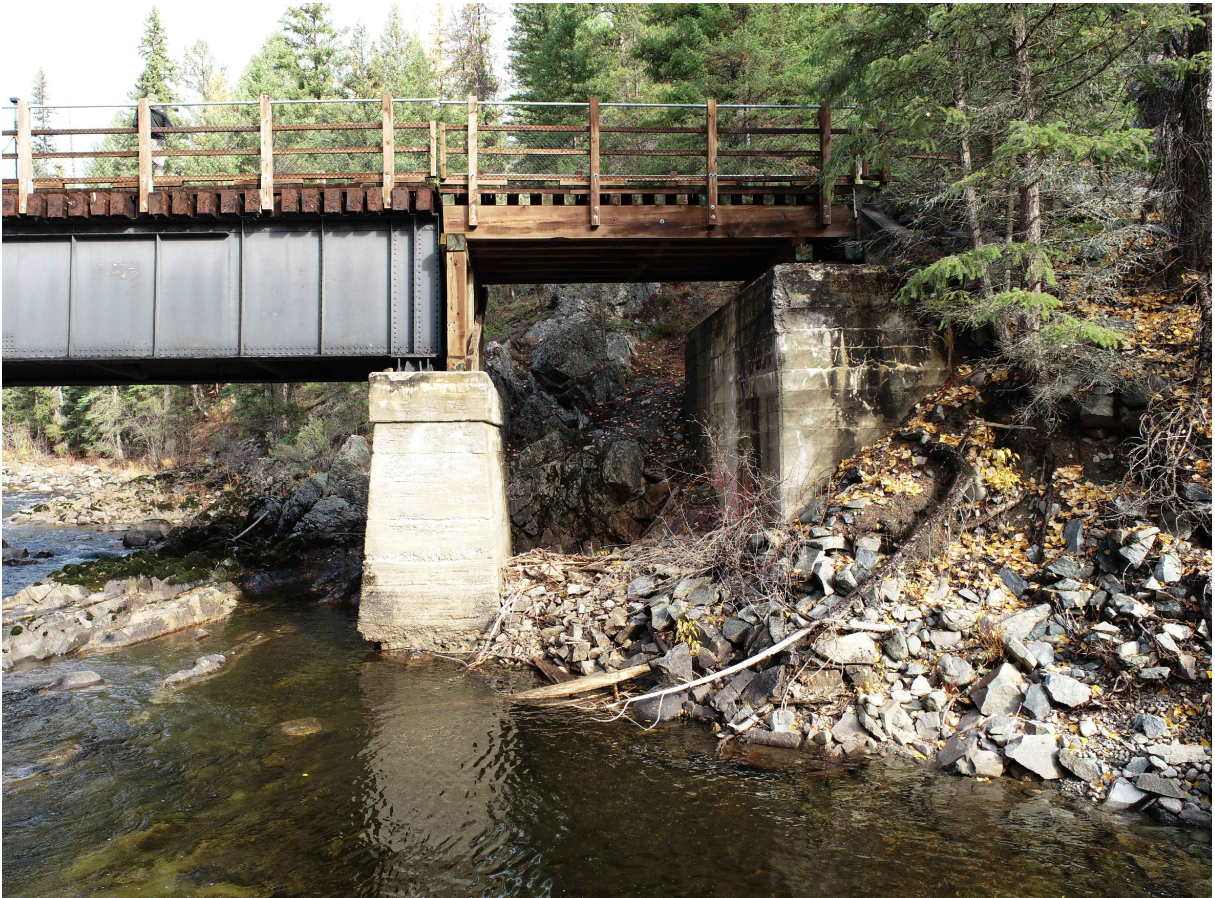
PHOTO 8: UNDERMINING AT THE DOWNSTREAM CORNER OF PIER
