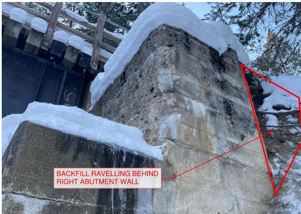
Figure 4-1: Backfill ravelling behind right abutment wall.
