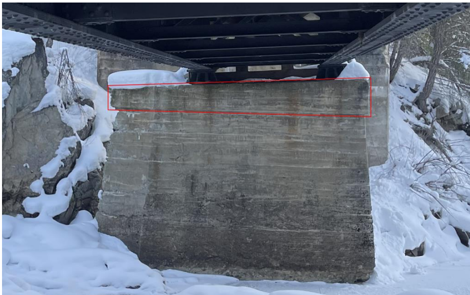
Figure 2-9: Varying pier cap thickness (looking at left bank). Bridge appears to be superelevated.
