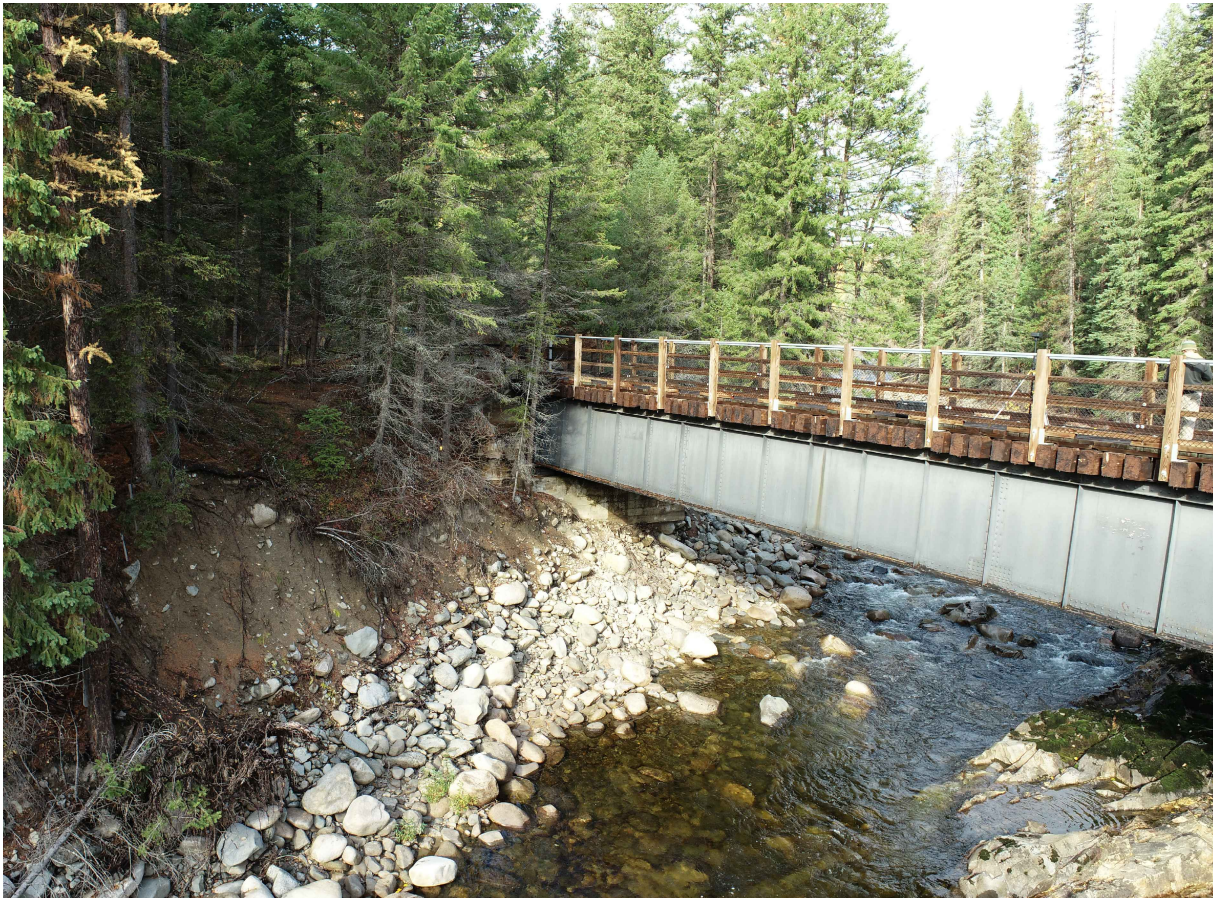
PHOTO 7: EROSION AT THE "RIGHT" BANK DOWNSTREAM OF BRIDGE
