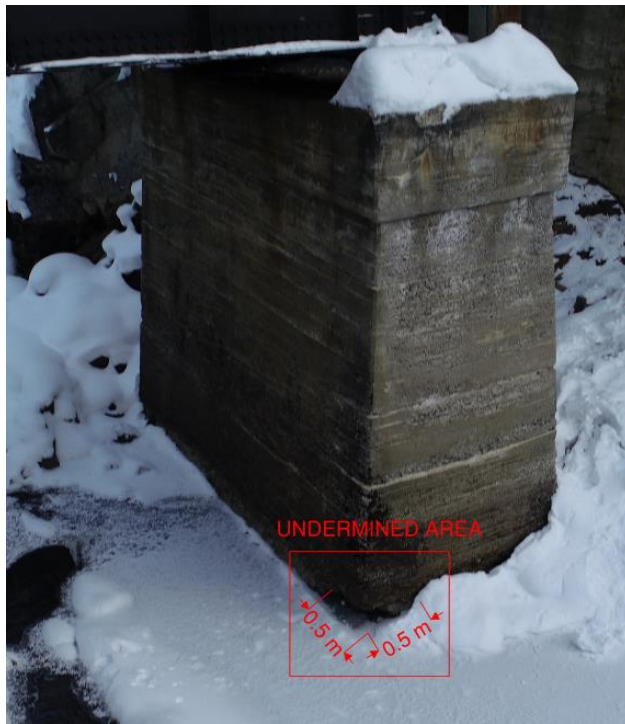
Figure 2-7: Approximate extents of undermined area at the concrete pier.
